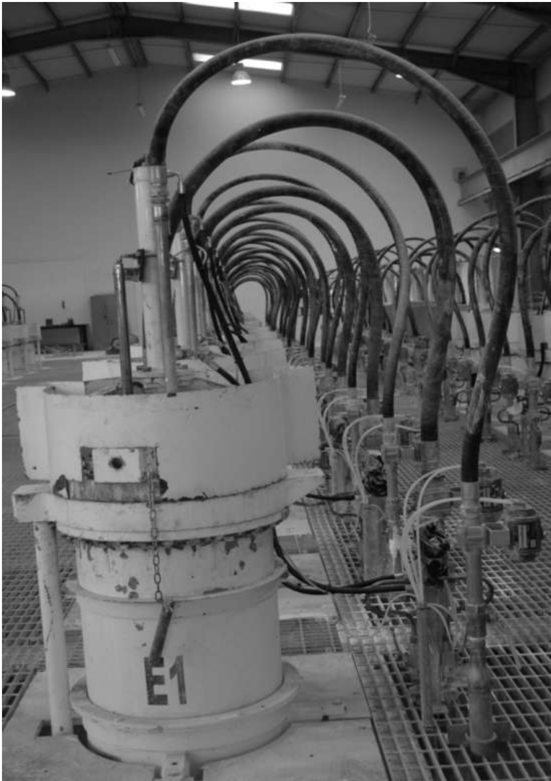
Hydraulic tube presses at Rock Dryer, Bugle.
